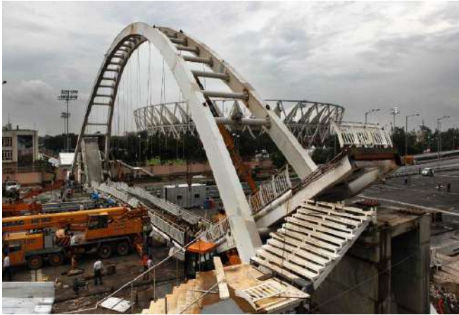
Fig. 1 Bridge collapse near Jawaharlal Nehru Stadium in New Delhi
