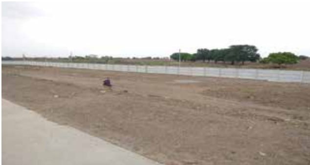
Fig.18: Mahasamruddhi express highway boundary wall by Smart Built Prefab Private Limited, Maharashtra [16]
