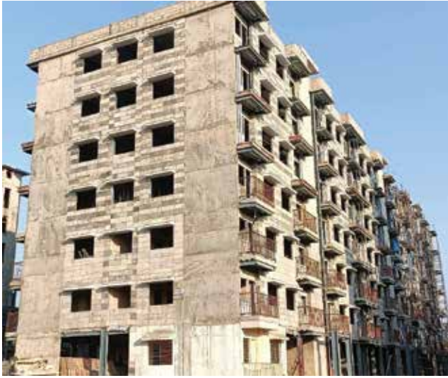
Fig.14: Placement of Precast Concrete Panels filled with Light Weight Concrete in LGS frames
