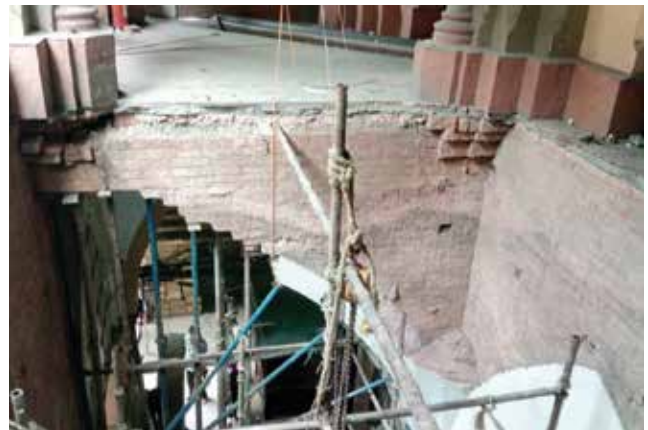
Fig. 9: Collapse of 1 st floor
