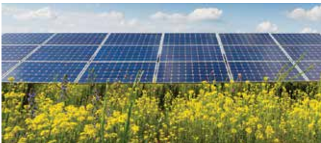
View of Pinnapuram Solar Panel Project
