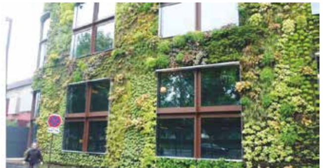
View of moss growing concrete
