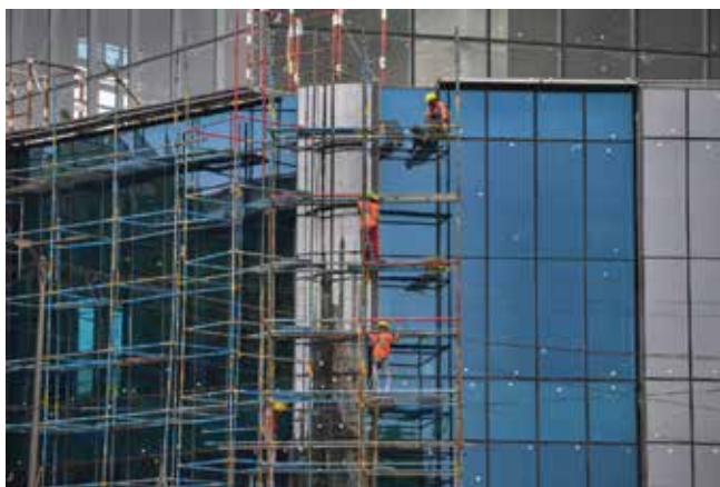
Expensive and inappropriate building materials only add to energy cost
