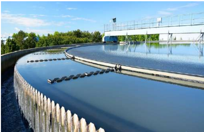
Fig. 2: Effluent Treatment Plant
