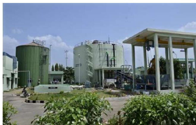
Biomethanation plant at Koyambedu market
