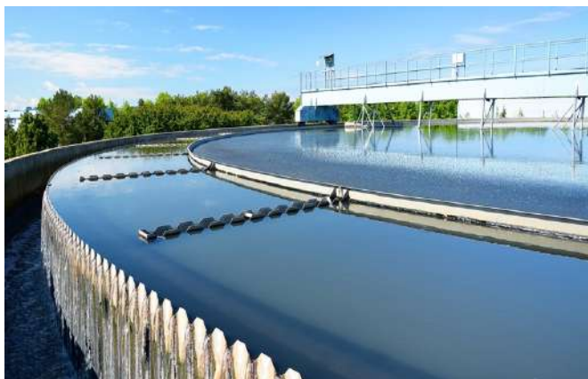
Fig. 2: Effluent Treatment Plant
