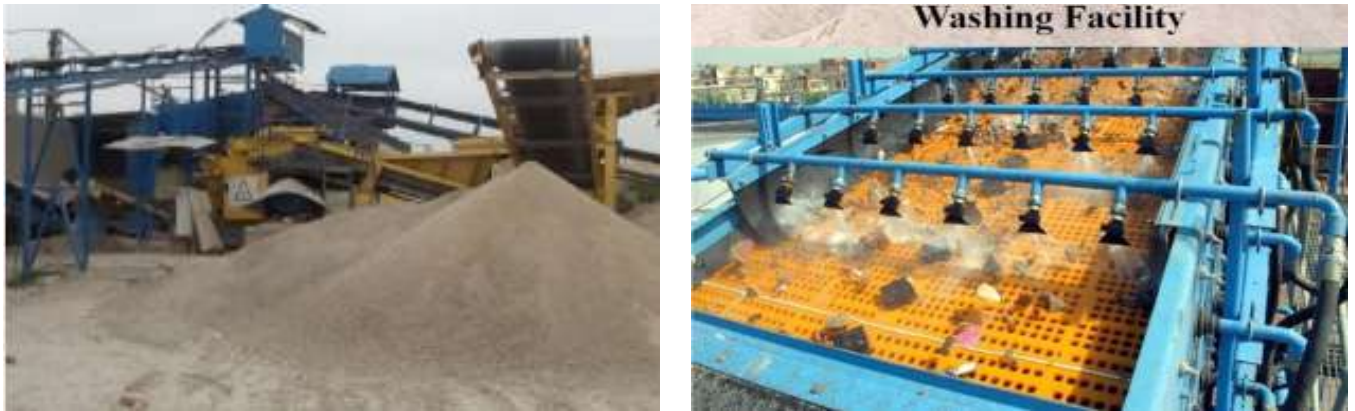
Fig. 2: Equipments installed at C&D Waste Facility at Burari
