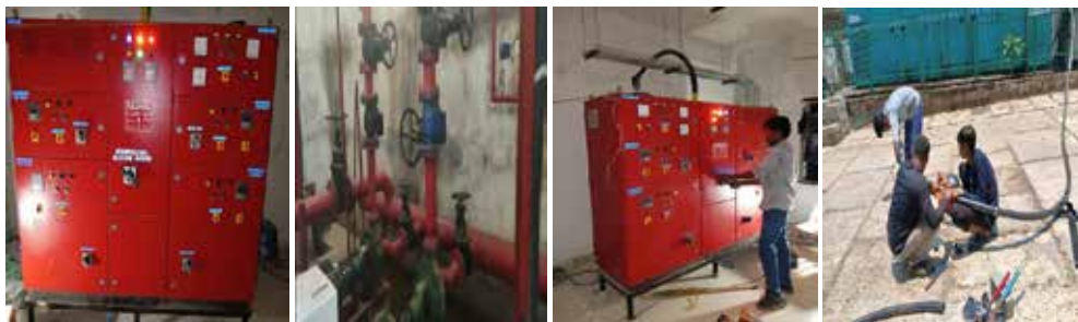
Fig. 2: Successful checking done after installation and connection of automated system controller to control the operation of the fire pumps
