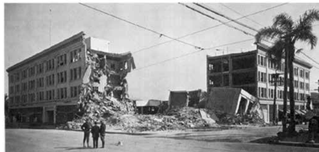
Fig. 5: Collapse of Re-entrant corner of the "L" shaped Building in 1963 Macedonia EQ, Skopje
